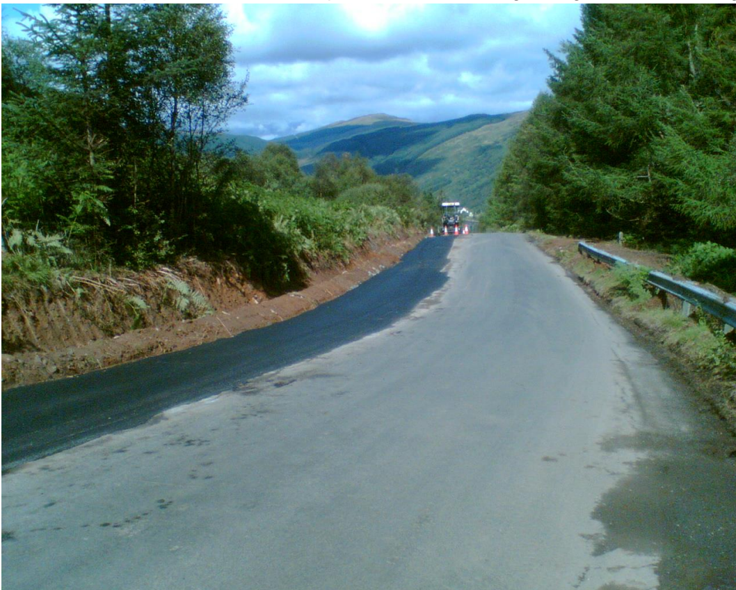
Widened pinch point, downhill lane, prior to final surfacing Craigendive 21 st August
