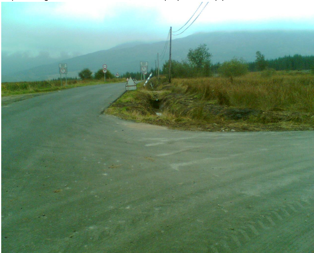
Top of Weight Restricted section, ditches prepared for pipe and ballast fill. 19 th Sept
